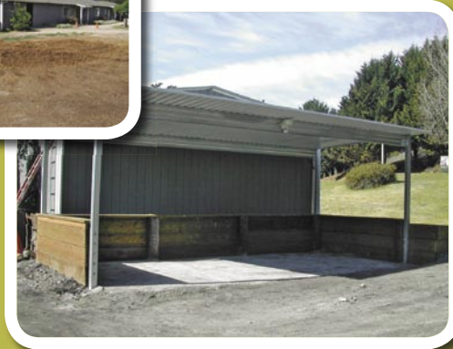
» AFTER: Covered manure bunker with concrete floor
